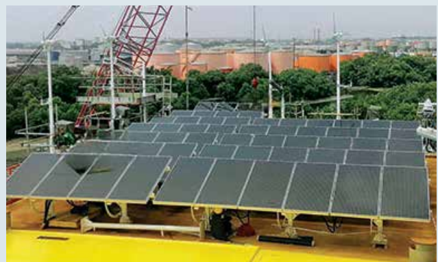
Solar Hybrid Wind Turbine installed and commissioned in one of the remote offshore Oil & Gas Platforms
