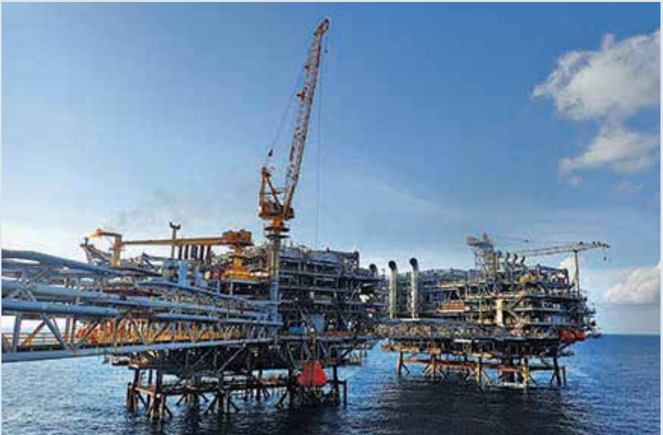
Offshore Crane, Guntong Delta Platform, Malaysia
