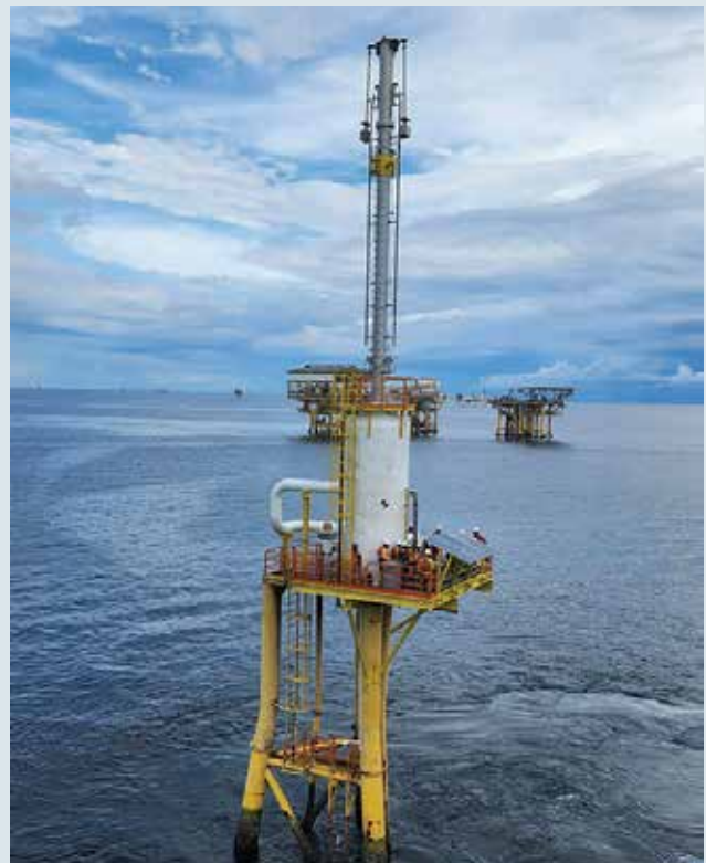
Advanced Flare System Installed and Commissioned to meet zero continuous venting directives by 2024 as per EP Flaring Venting Framework
