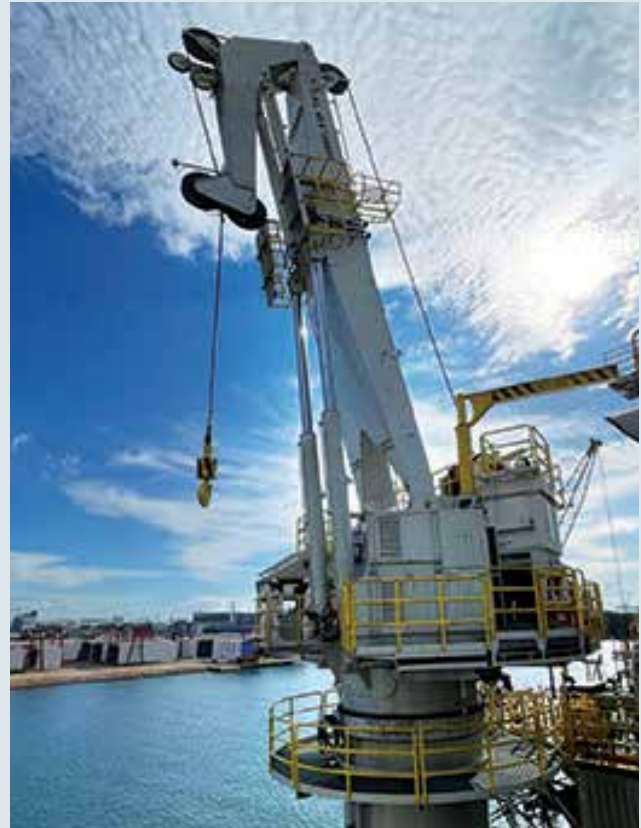
Offshore Crane, Golar GIMI FLNG, West Africa
